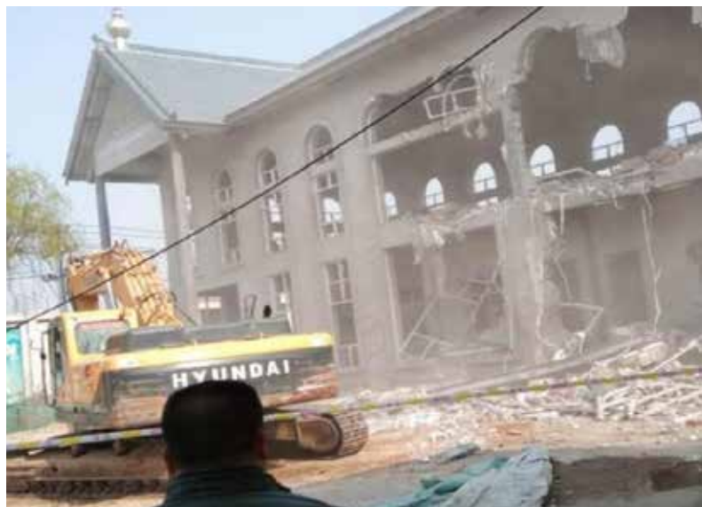
A newly constructed convent being torn down in Northeast China. Photo by an unknown Chinese believer.
