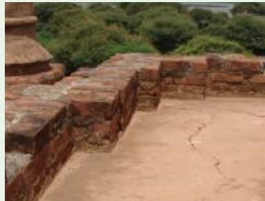
Cracks in the roof of a temple, Bagan, Myanmar, 2016. Photo: Eugénie Crété.
