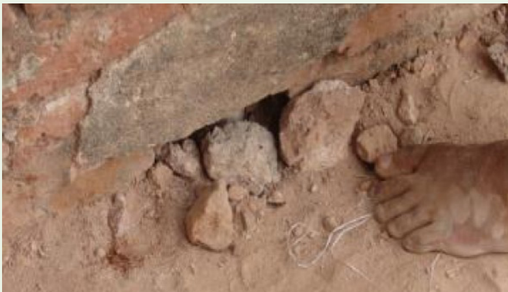
Holes in the roof waterproofing system of a pagoda in Bagan, Myanmar, 2016. Photo: Eugénie Crété.
