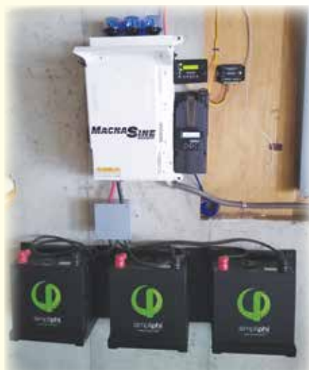
Inverter and batteries for a local off-grid installation.
