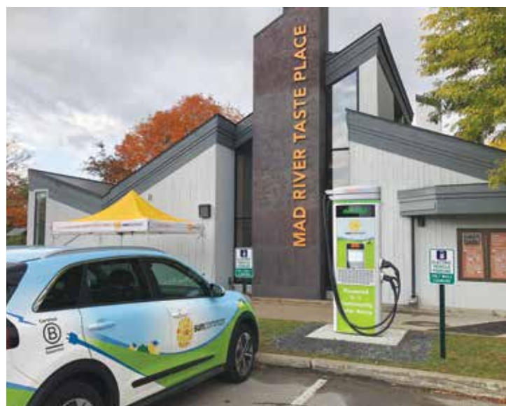
A super-fast charger was installed by SunCommon at Mad River Taste Place in Waitsfield, VT. It has a capacity of 62.5 kilowatts, which can charge many EVs in half an hour. The power for the EV charging station is provided from a community solar array. Image: Mad River Taste Place.
