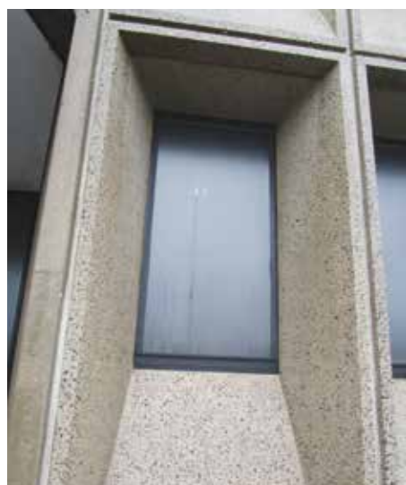
Concrete panel façade with existing windows prior to retrofitted construction. Courtesy photo.
