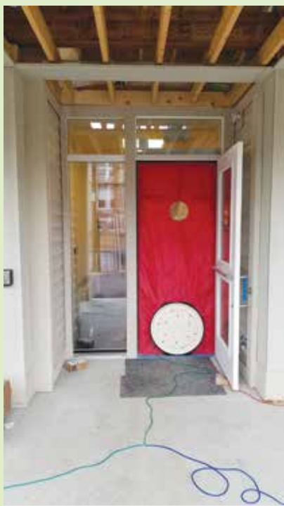
Blower door testing is done to assure that the building meets the high-efficiency standards.
