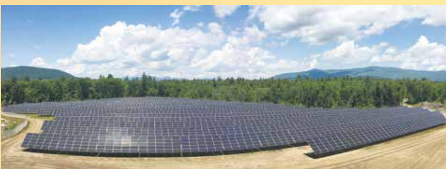
A 2.0MW solar array consisting of 8000 panels is located on land owned by NHEC off Moultonborough Neck Road in Moultonborough, NH. Power produced by the array will enter NHEC's distribution system at nearby Moultonborough Neck Substation. Image: NHEC.
